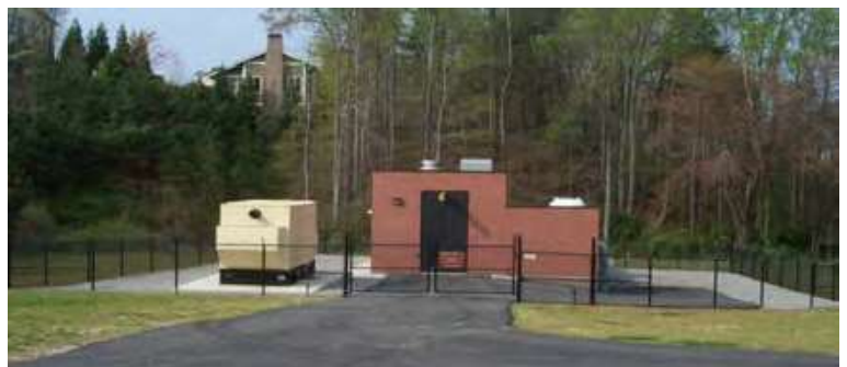
Department of Water Resources Lift Station
